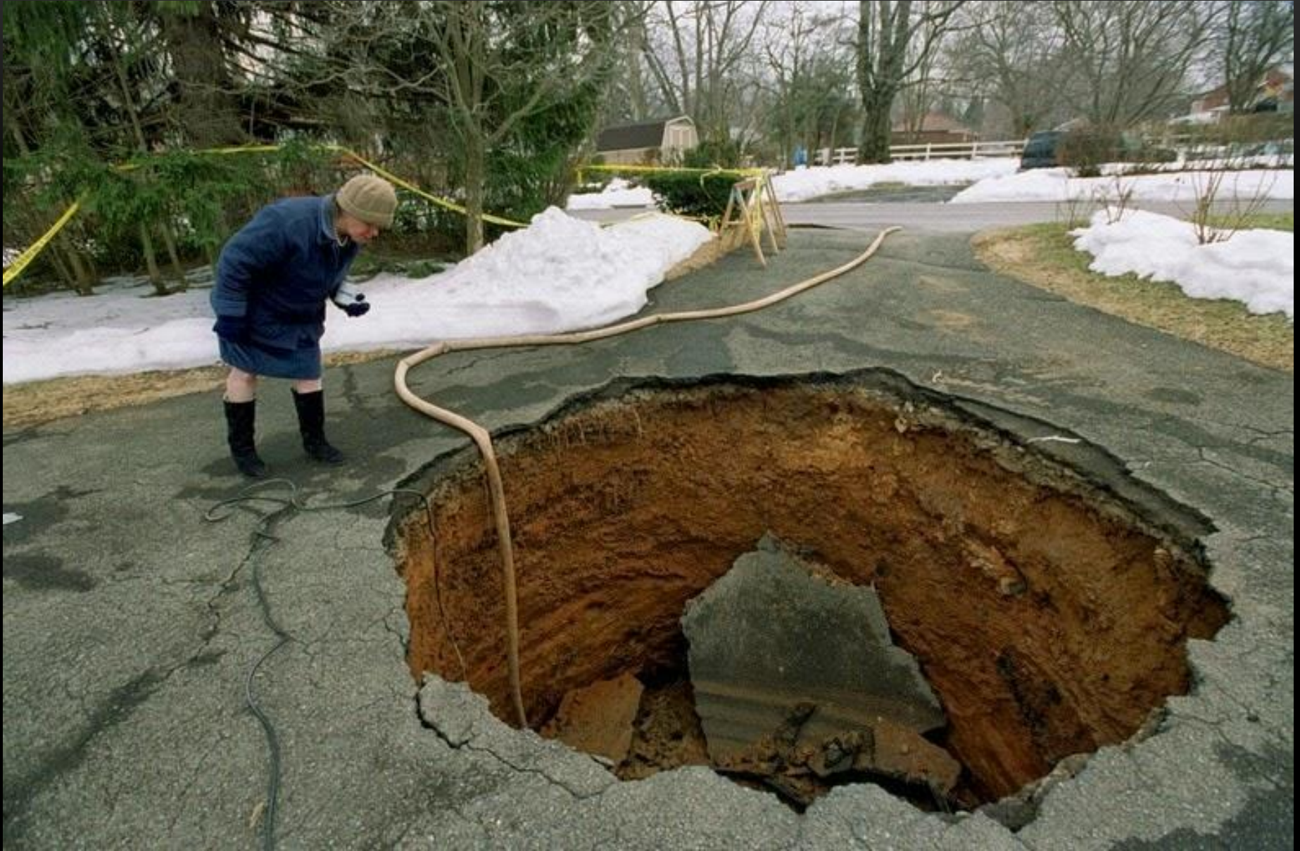
Locheam sinkhole, Baltimore Sun newspaper (2013)
